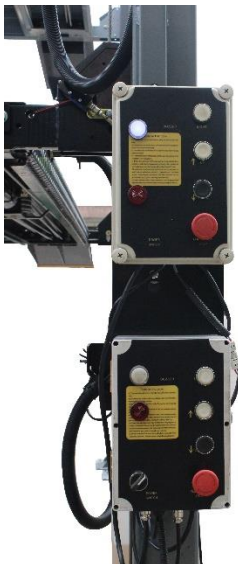
Dual control boxes
